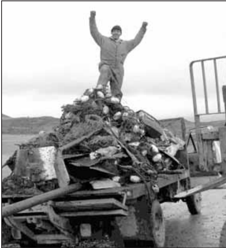
Crew member Edward Saul Blatchford stands on a truck load of debris removed from the Unalakleet Slough.
